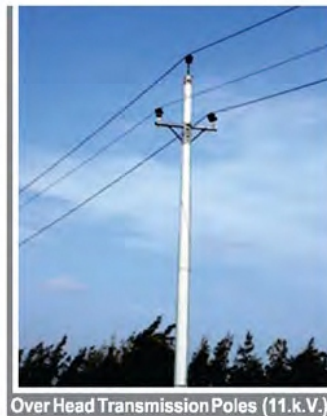
Over Head Transmission Poles (11.k.V.)
