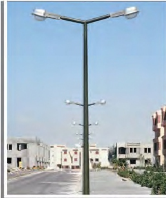
Street Lighting Poles
